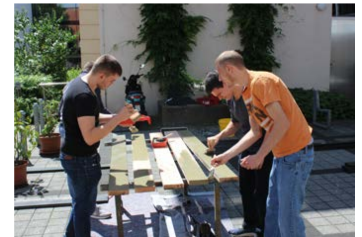
Twelve park benches at St. Nikolai were restored by our trainees to their former splendour.
