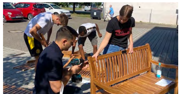
Thanks to the craftsmanship of our trainees, the seating area for the elderly in Efringen-Kirchen is taking shape.
